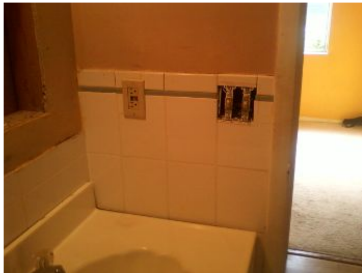
Light switch cover missing
