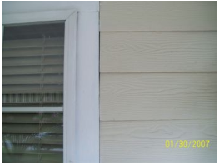
Window needs caulking
