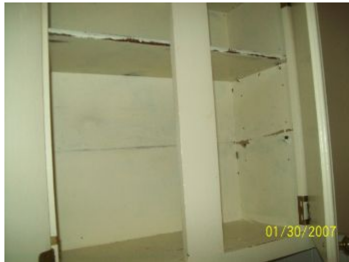
Shelves missing from cabinets
