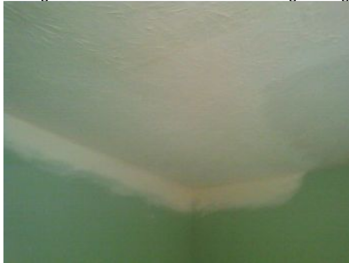
Sign of previous water leak
