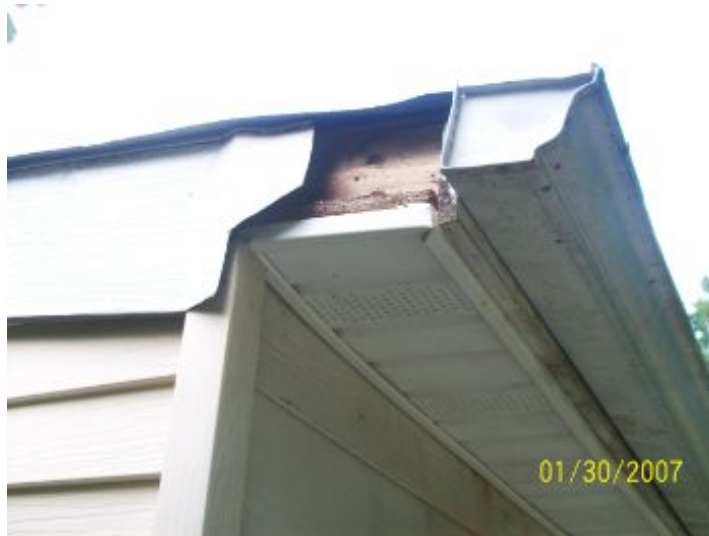
Fascia is missing- wood is damaged
