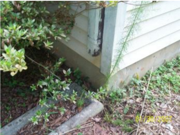
Downspout missing section
