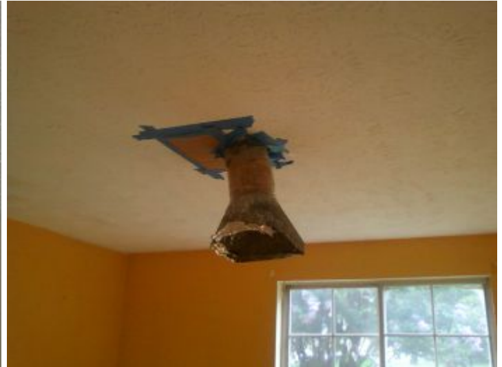
Ceiling damage- no vent cover
