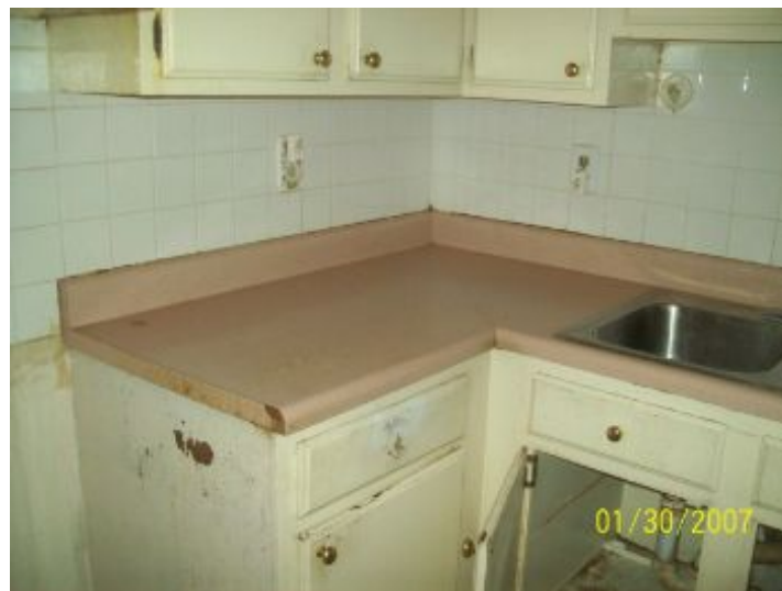
Laminate counter top is damaged.
