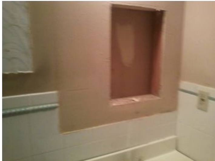
Mirror and medicine cabinet missing
