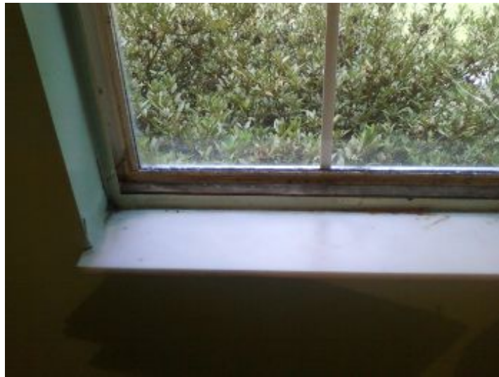
Black mold on window frames
