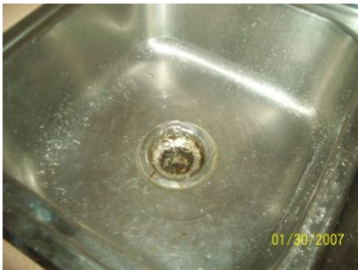
Sink is clogged
