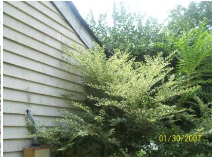
Gutters are missing on rear of house
