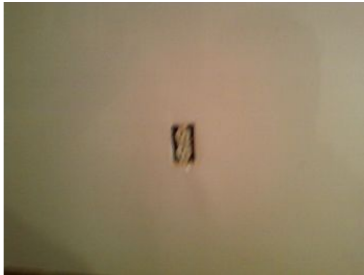
Outlet cover is missing
