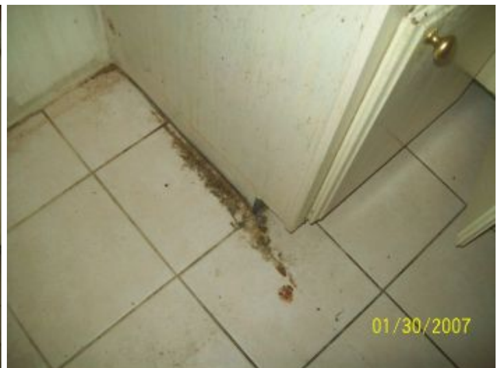
Mold on and around cabinets
