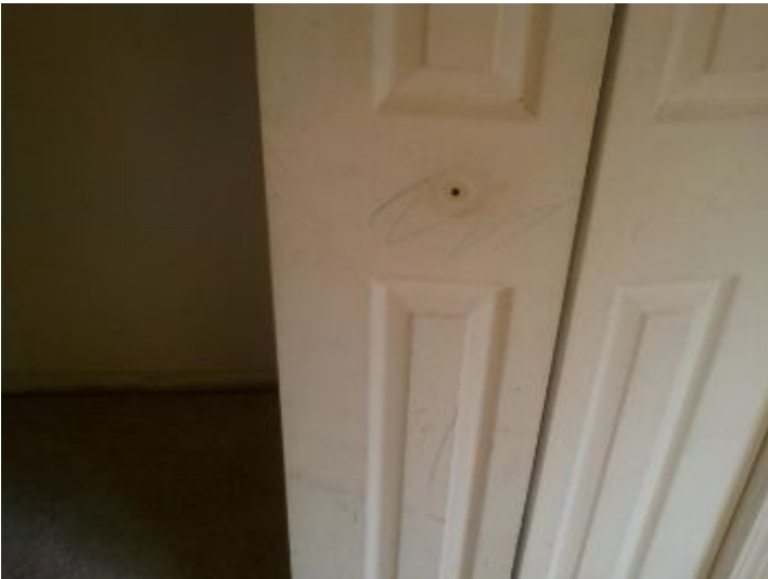
Several handles missing from closet doors
