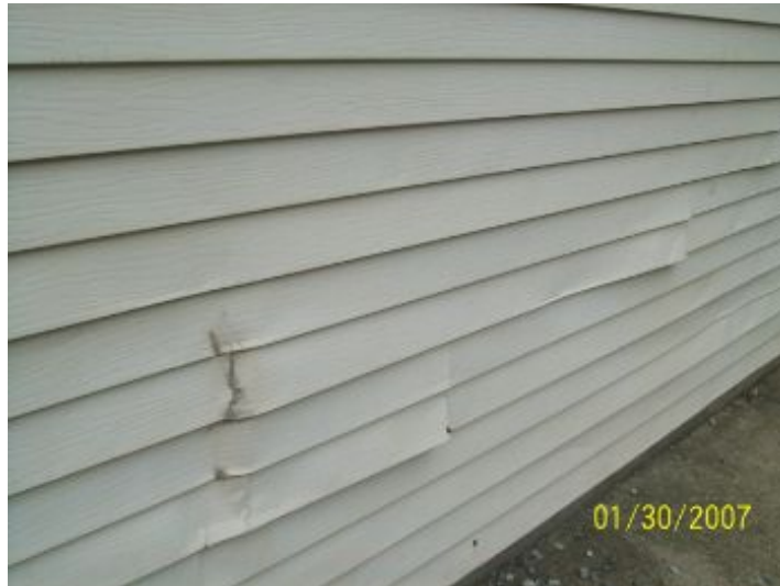
Aluminum siding is damaged in several places
