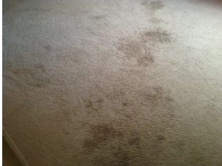
All carpet is worn and stained
