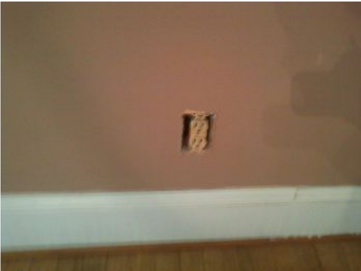
Missing outlet cover
