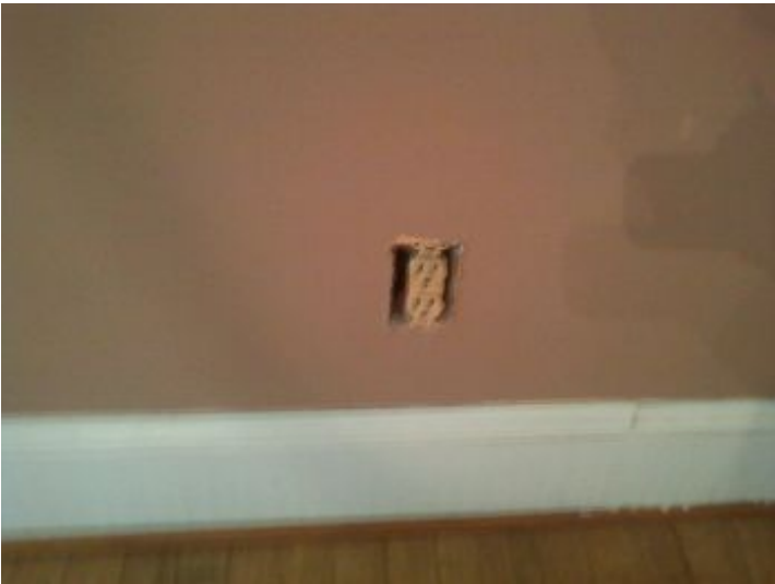
Missing outlet cover
