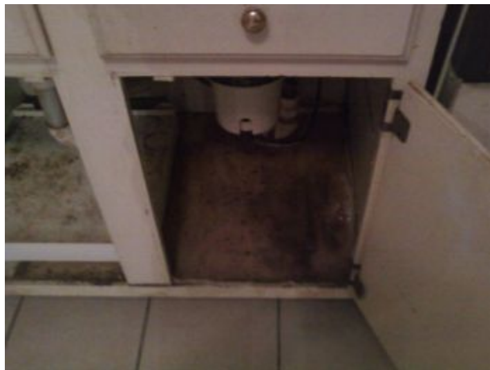
Disposal does not operate
