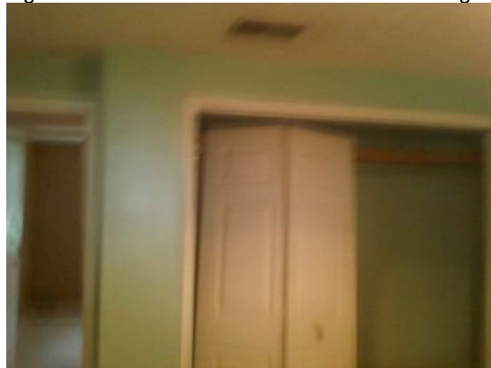
Doors not mounted
