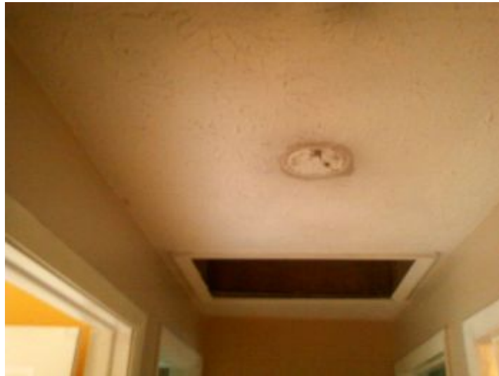
missing smoke detector
