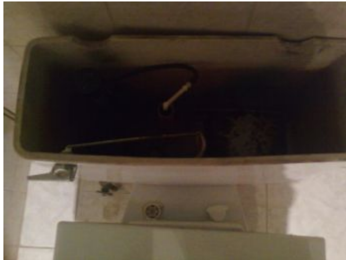
Moldy toilet does not operate
