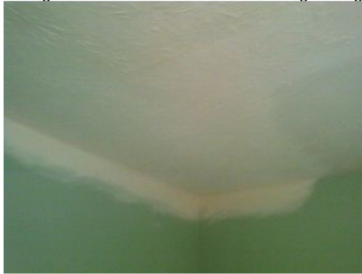
Sign of previous water leak
