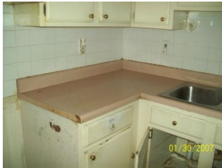
Laminate counter top is damaged.
