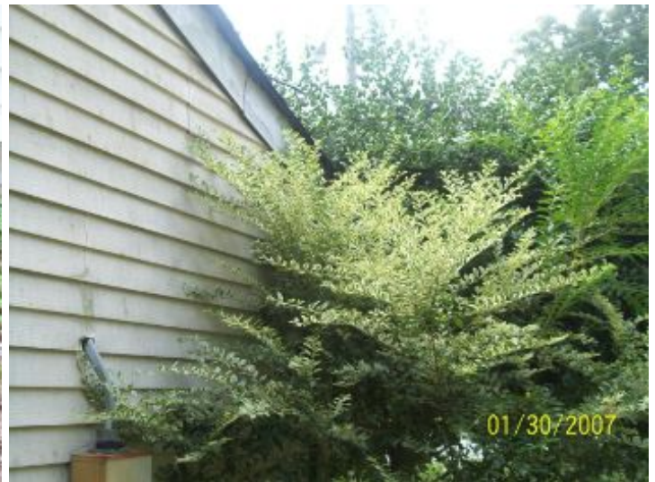
Gutters are missing on rear of house
