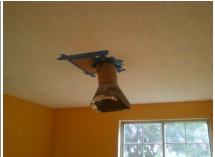
Ceiling damage- no vent cover
