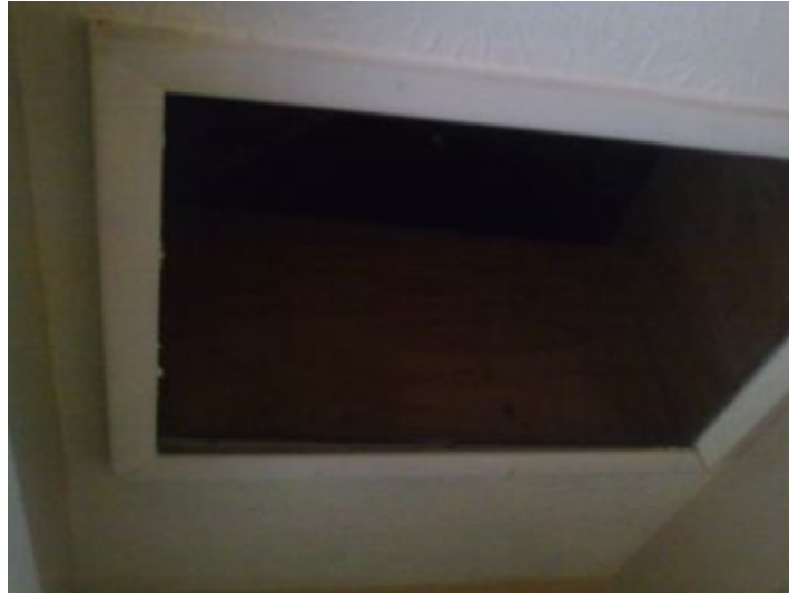
Missing scuttle hole cover
