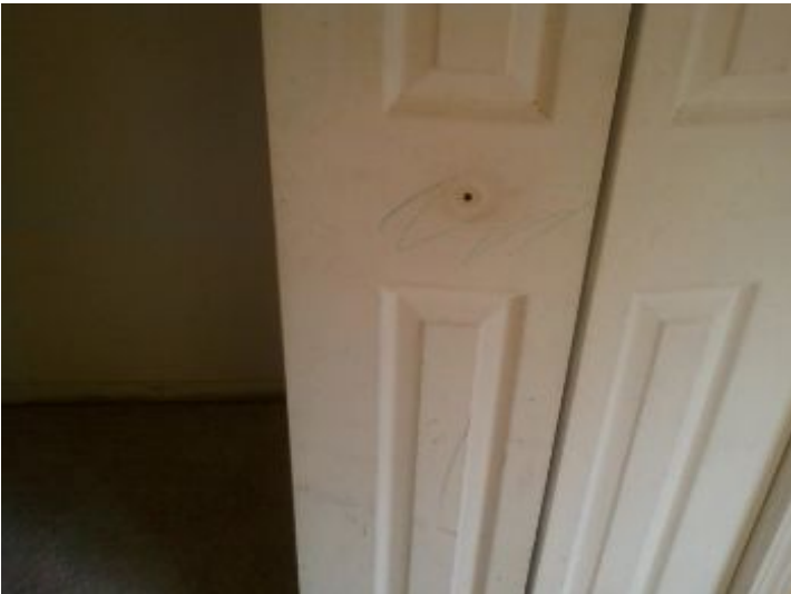
Several handles missing from closet doors
