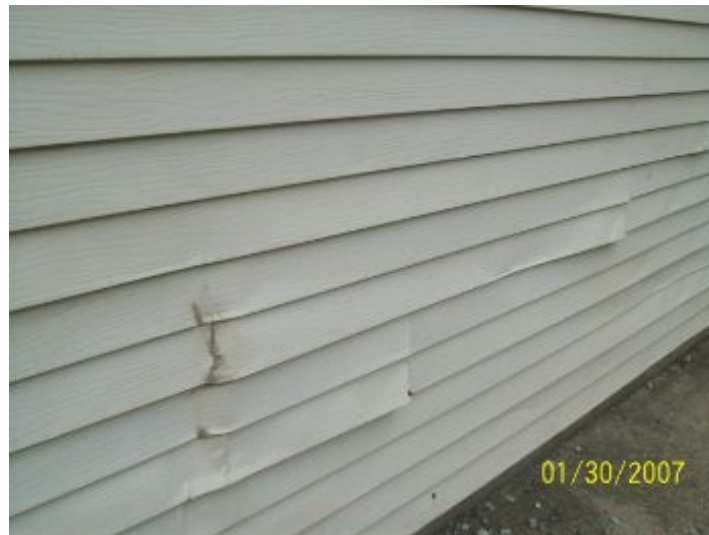
Aluminum siding is damaged in several places
