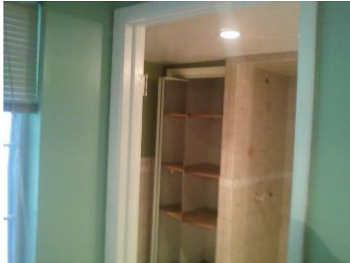
Door is missing
