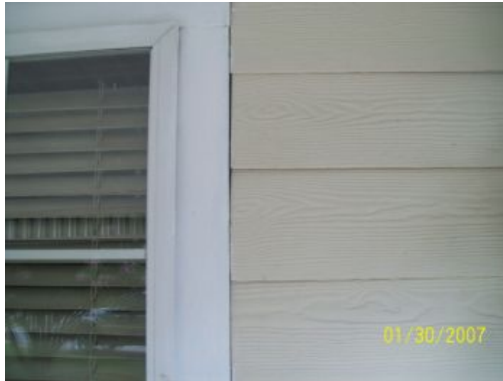
Window needs caulking
