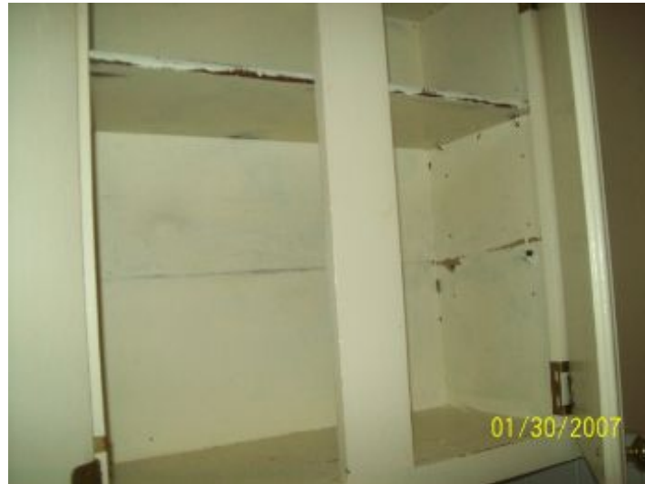
Shelves missing from cabinets
