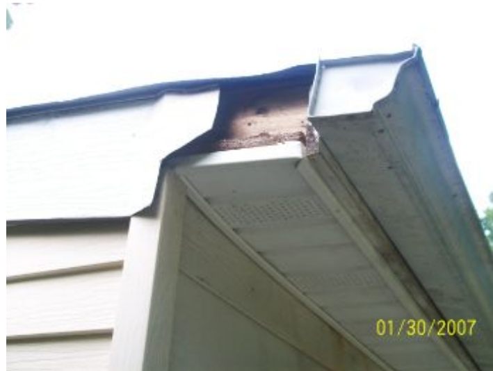
Fascia is missing- wood is damaged
