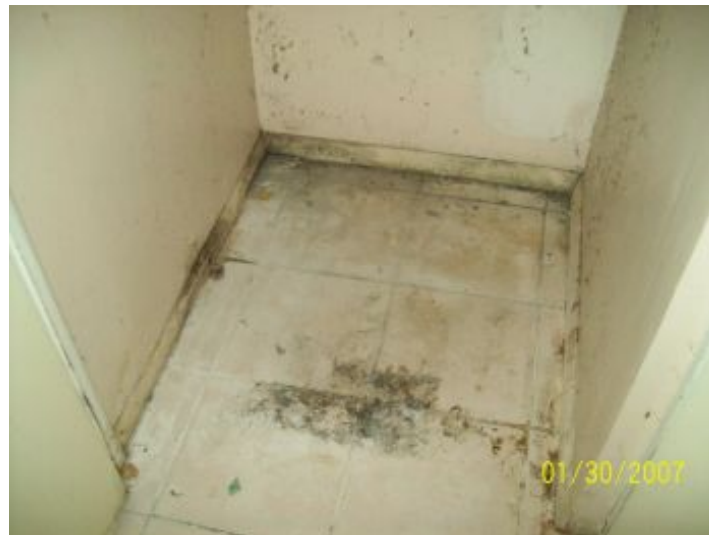
Black mold in laundry closet
