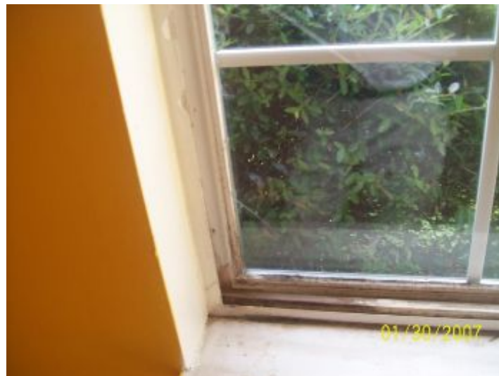
Several broken window panes
