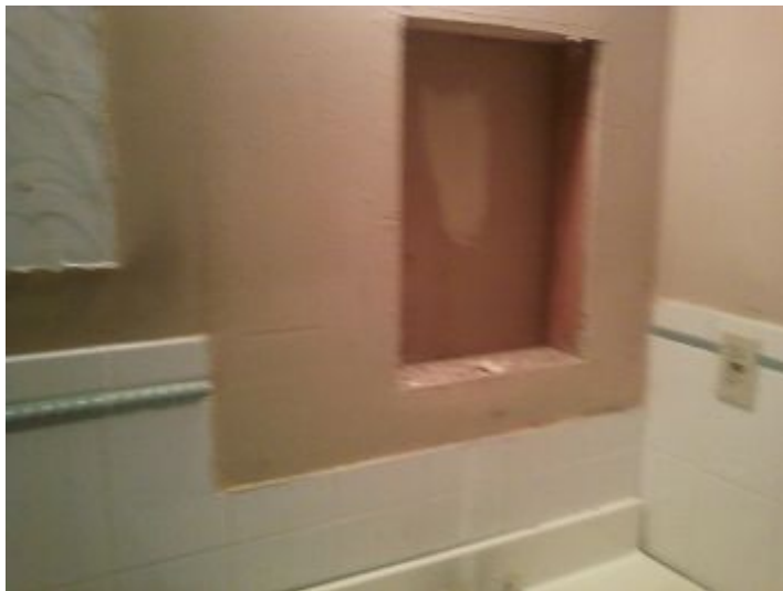
Mirror and medicine cabinet missing
