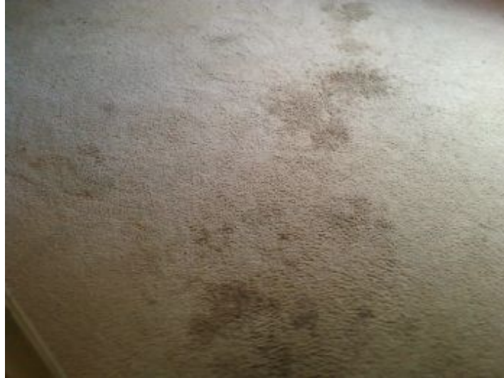
All carpet is worn and stained
