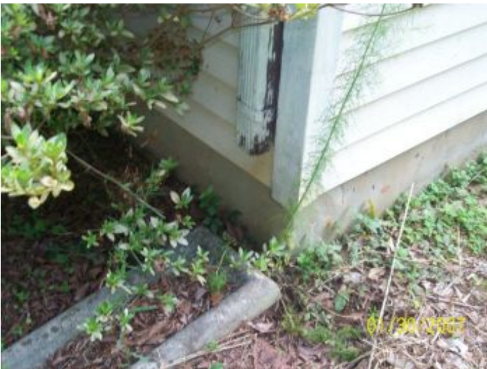
Downspout missing section
